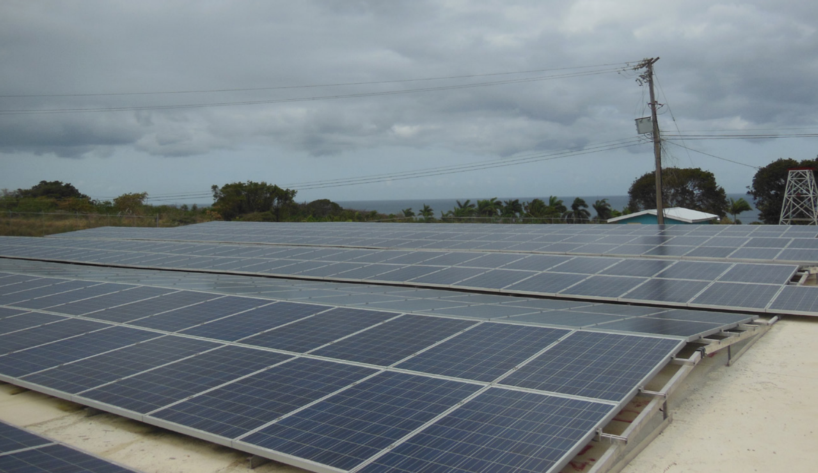
> Solar powered BWA pumping facility, St. Peter
