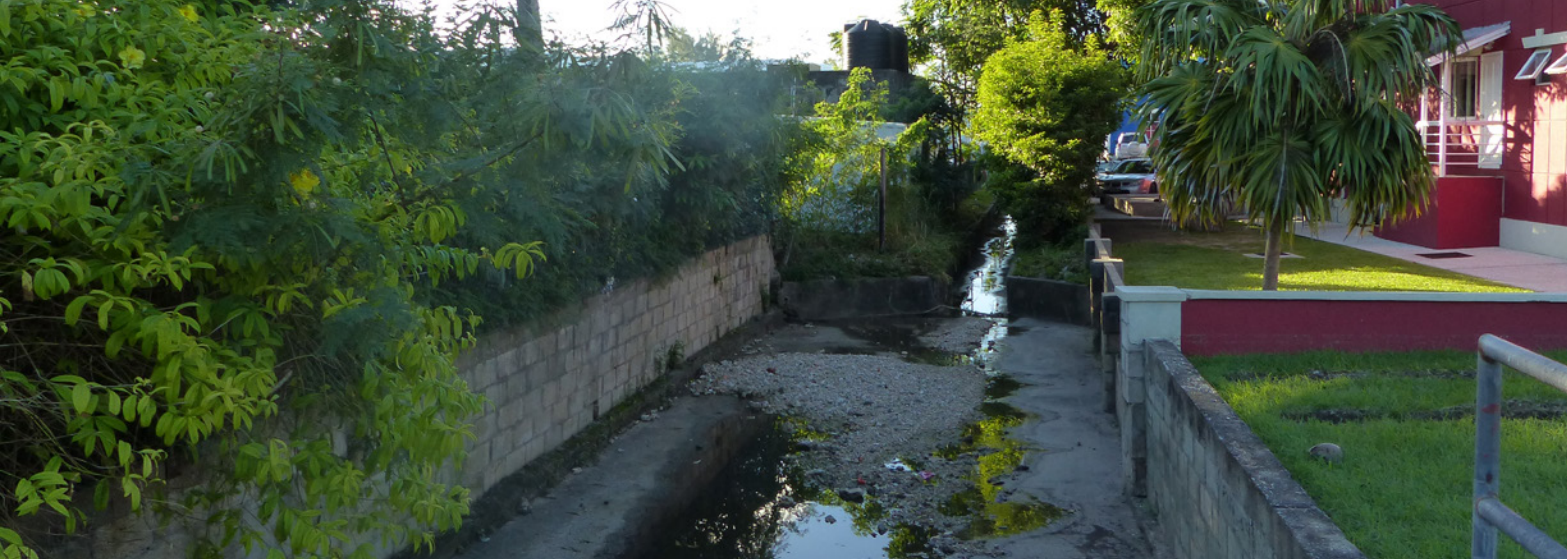
> Channelised gully outfall prone to flooding
